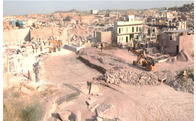
Fig. 4: Due to automated procedures including drilling, crushing, screening and blasting, etc., noise level is much higher than the recommended limit. Moreover, Workers who use pneumatic tools like drills can get vibration illnesses.
